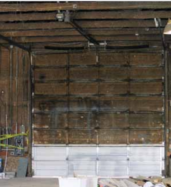
THE SCENE OF THE ACCIDENT: This is the 16' x 16' garage door and the trolley operator involved in the accident. The two replacement sections had been installed a week earlier. (Photo used with permission.)
