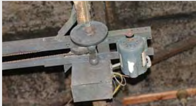
THE OPERATOR INVOLVED: This operator, thought to be 30 years old, is missing its belt because it had burnt off during the accident. (Photo used with permission.)
