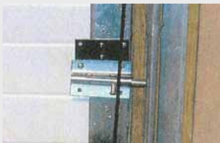
THE LOCK: This slide lock, installed by Cort, was thought to be involved in the chain of events that led to the accident. (Photo by Dynamic Evidence of Fort Lee, N.J. Used with permission.)
